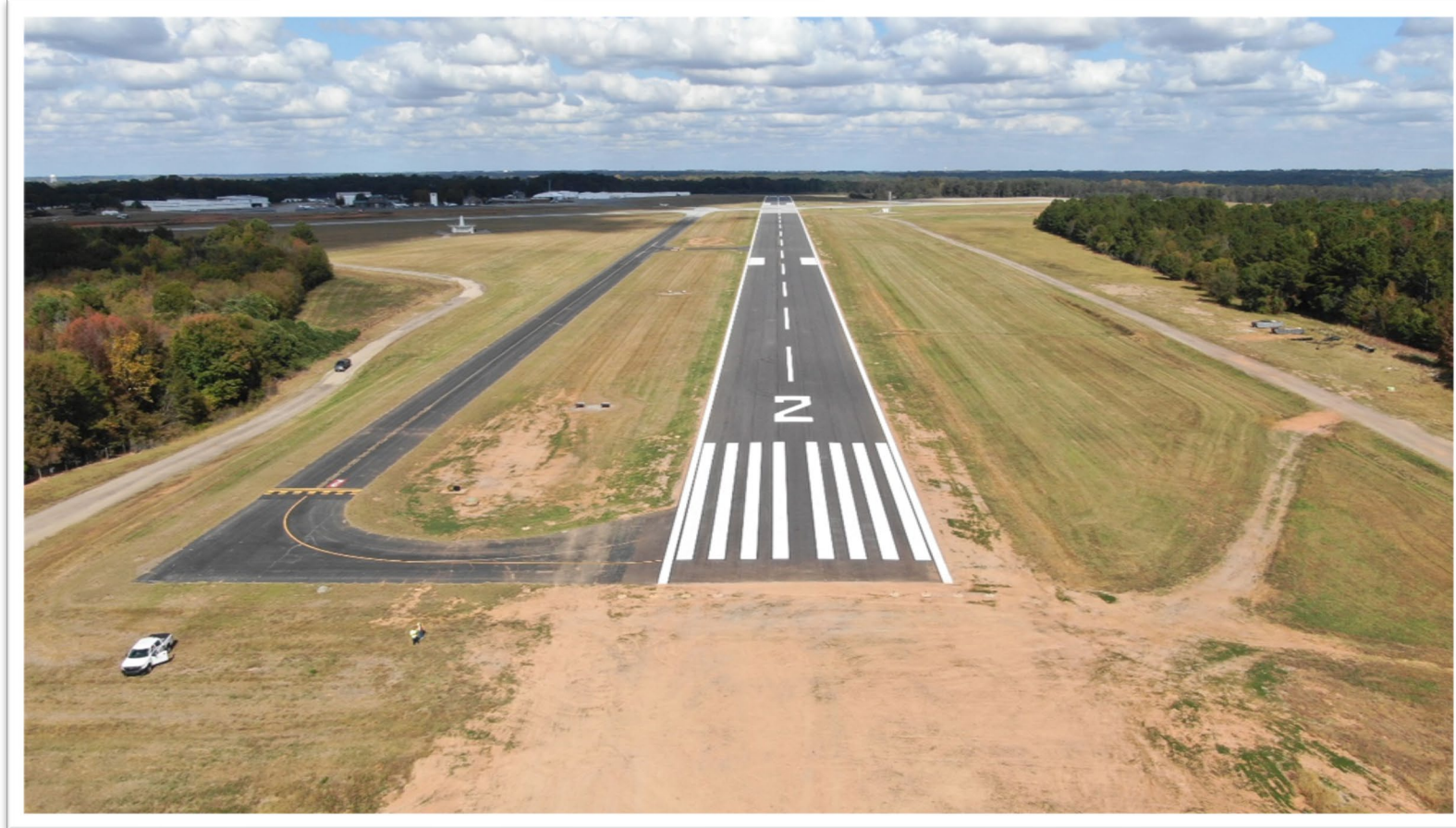
Athens – Ben Epps Airport Reconstruction of Runway 2-20 and Safety Area Improvement Total Project Cost: $4,701,744
