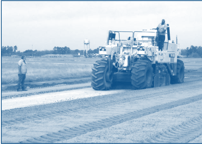
Contractors work at the Waycross-Ware County Airport to prepare the reclaimed base and existing surface course on Runway 5/23 for paving.
